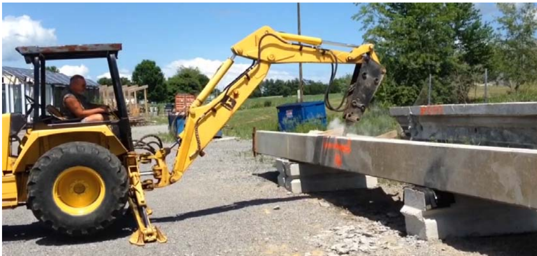
Figure 4-3 – Hydraulic Breaker Damaging Strands
