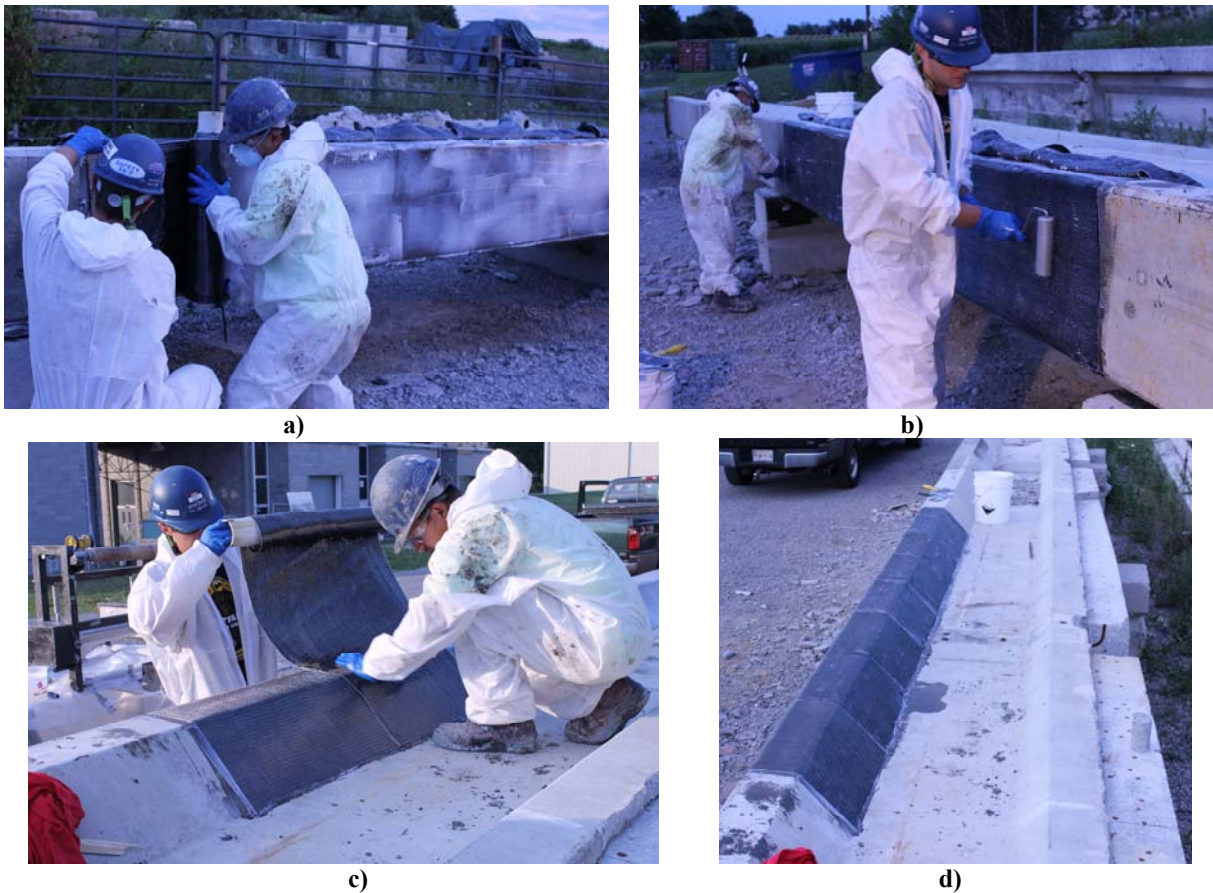
Figure 4-22 – FRP Sequence of Application a) Steps 1 b) Step2 c) Step 3 d) Completed Repair
