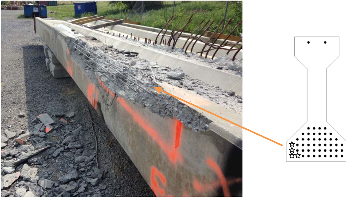
Figure 4-4 – Damaged Prestressing Strands
