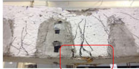
G1-2-FRCM (slippage in PBO)
