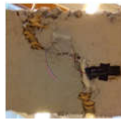
Slippage in PBO
